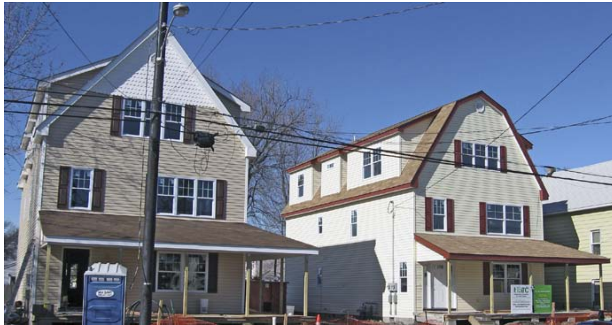
Interfaith Neighbors is finalizing construction on two two-family homes at 47 & 51 Ridge Avenue. These homes represent our 22nd & 23rd affordable housing projects!
